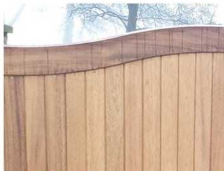
This gate has been treated with preservative but not with Oil. The water is soaking into the top of the gate.
