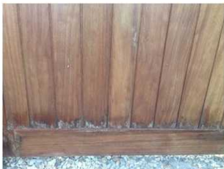
This gate has been poorly maintained. Water has ingressed and started to damage the gate.
