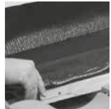
Stretch lead replacement roll to shape if necessary and press to fit snugly and securely over all surfaces.
